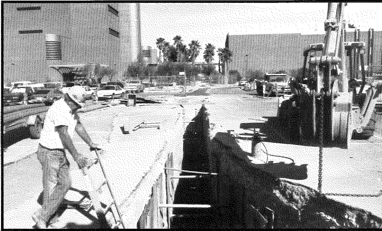
Digging Trenches: The UA's new underground communications system requires massive construction across campus, such as the digging of a trench between the Electrical and Computer Engineering building and the Harvill building.
